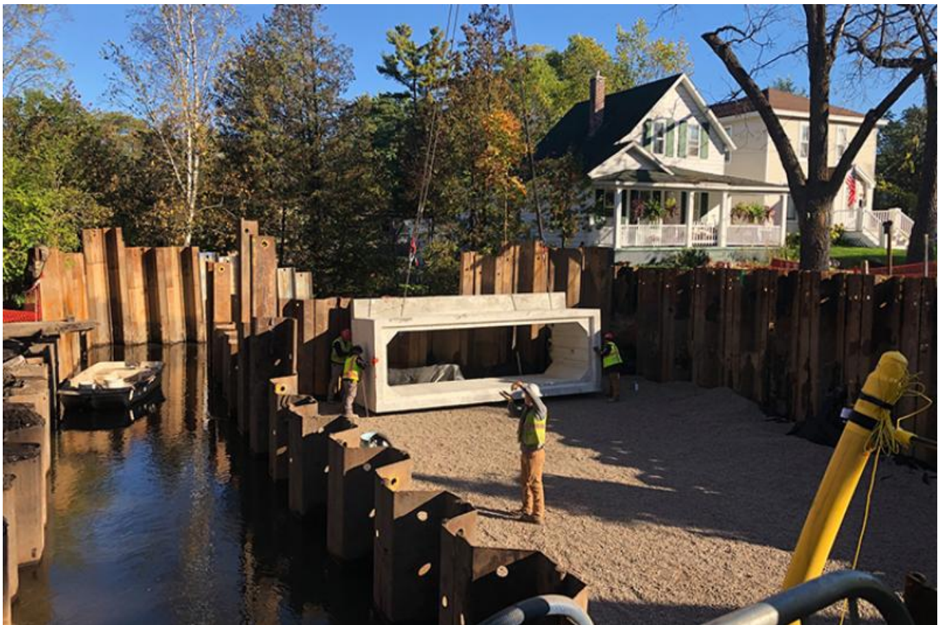
Culvert replacement underway on Kids Creek. Credit: Zach Cole/City of Traverse City.
