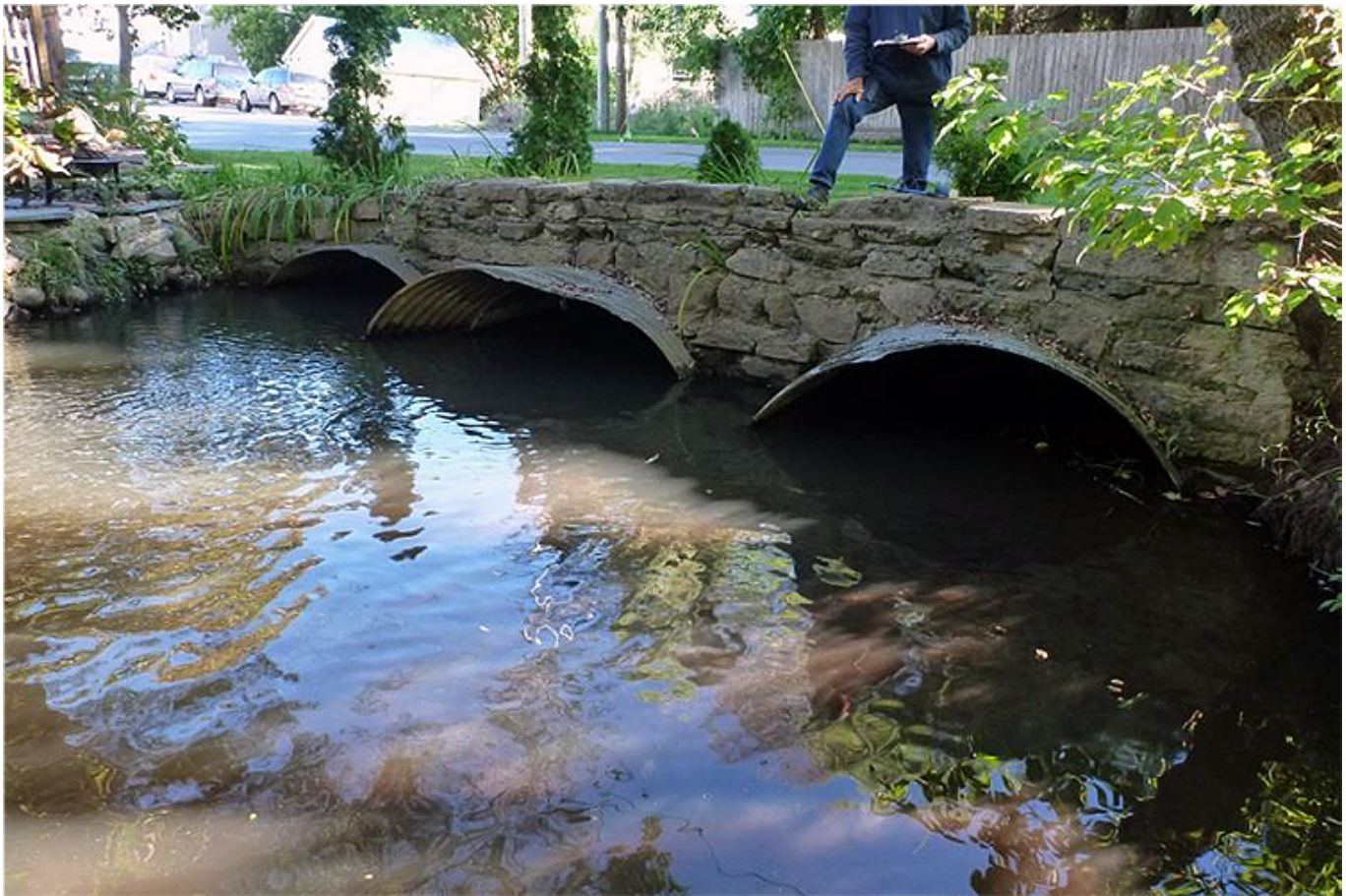
Undersized culverts on Kids Creek, prior to restoration. Credit: The Watershed Center Grand Traverse Bay.
