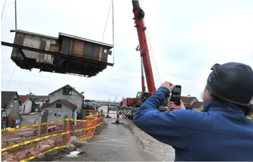
David Kareck, owner of the Village Cheese shanty, takes video of the shanty being lifted by crane off Leland's Fishtown docks and placed in the nearby marina parking lot. The waterlogged and rotting foundation will be replaced and the shanty will return to its site by April. (Photo: John L. Russell, Special to The Detroit News)
